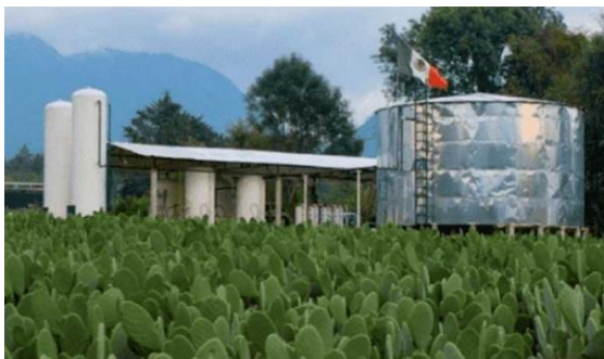
Nopalimex plant in Michoacán.
